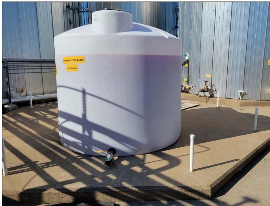
Figure 6: An Existing Pad in Tank Farm Designated for Wastewater and Distillation Products
